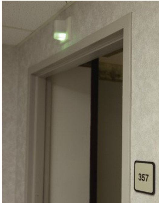
FIGURE 21-20 Light above the room door.
